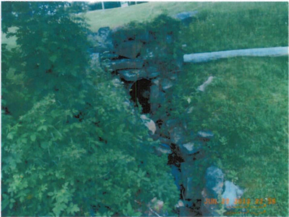
PA-4: Outfall which directs drainage from the south side of Pascal Ave. and to outfall PA-1.
