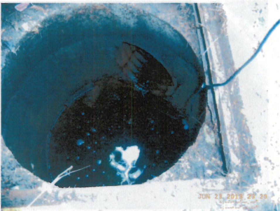
PA-4A: Catch basin on east side of Pascal Ave. at the corner of Ship Street and Pascal Ave. which flows towards PA-4.
